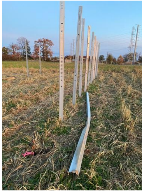
Figure 4. A damaged post (C-channel) as a result of hitting an underground rock during installation. A new post was installed after an 18-inch hole was augered into the ground and filled with compacted aggregate. Photograph by A.J. Both.
