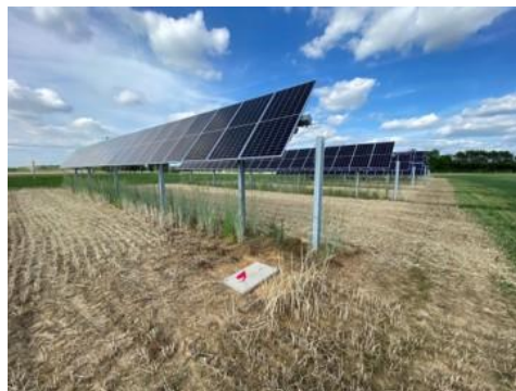
Figure 6. In-ground conduit connector box that was installed in an inconvenient location with respect to farming operations. Photograph by A.J. Both.
