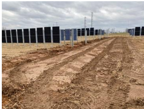
Figure 5. Example of the impact of equipment movement on the soil surface after a heavy rain event. Photograph by A.J. Both.
