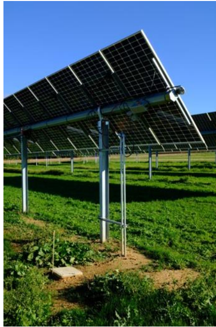
Figure 7. Conduit riser that was installed some distance away from a support post because the manufacturer claimed that underground conduits installed along the post would adversely impact the post's wind uplift strength. Photograph by A.J. Both.
