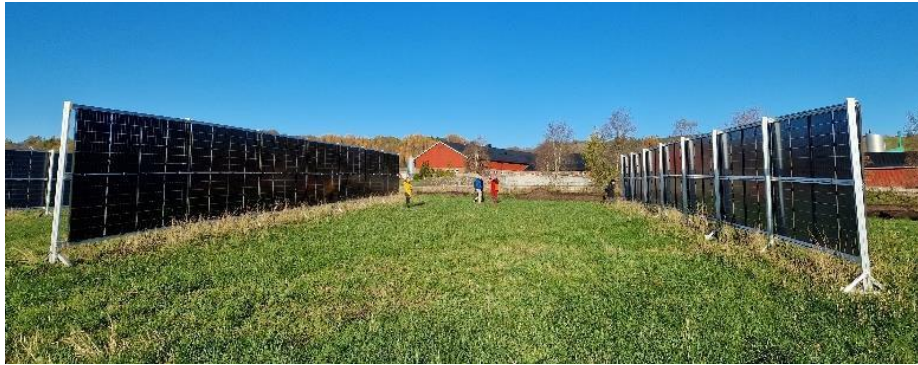
Figure 1. The 48 kWp AVS at Skjetlein High School.
