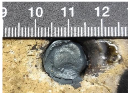
Figure 3. A damaged steel screw after exposure, with a numerical ruler for size identification
