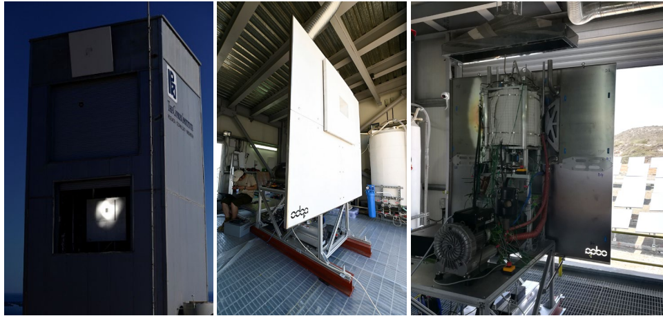
Figure 4. Odqa 10kW-scale solar thermal receiver installed on PROTEAS solar tower.
