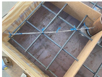
Figure 5. Thermocouples embedded in heat-resistant concrete slab
