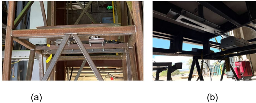
Figure 8. (a) load cells under test bin platform. (b) slide gate and actuator under furnace
