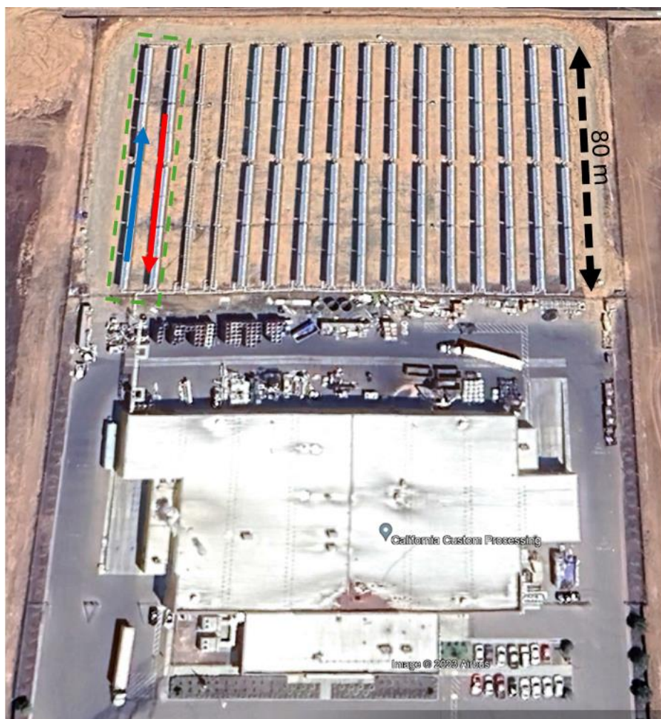
Figure 3. Pressurized water circulates in the solar field comprised of eight collector loops. The collectors are aligned in the north-south direction. The dashed green box highlights one of the eight parallel loop, showing the flow direction within the loop. Each loop can be seen to include four collectors in series. A scale is indicated to the right of the solar field.
